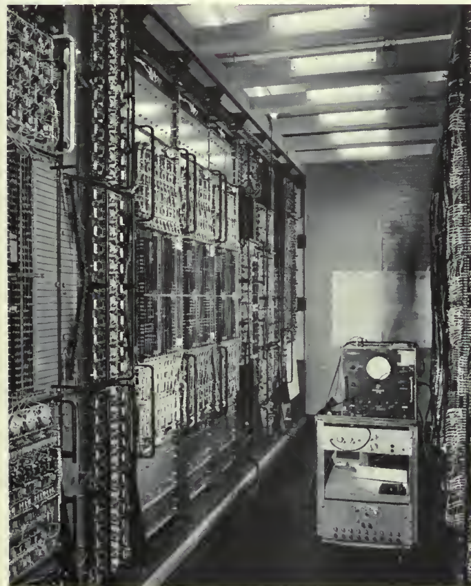
Fig. 5. View of central control.
